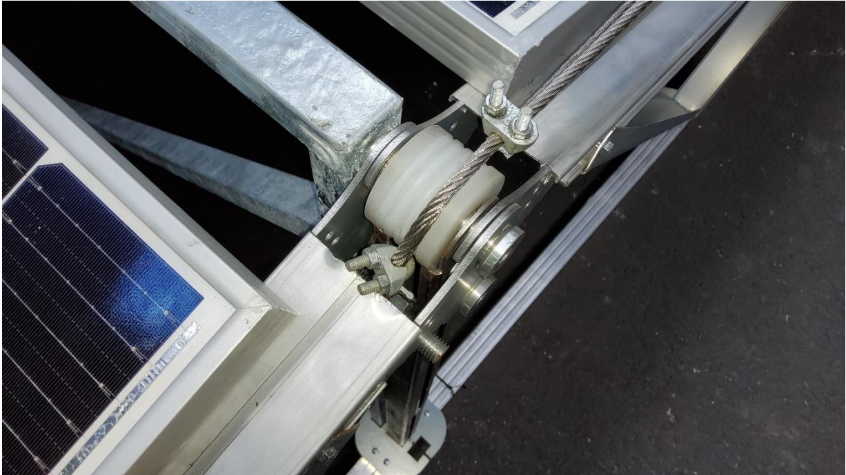
Fig. 2 Sample wire rope connection.
